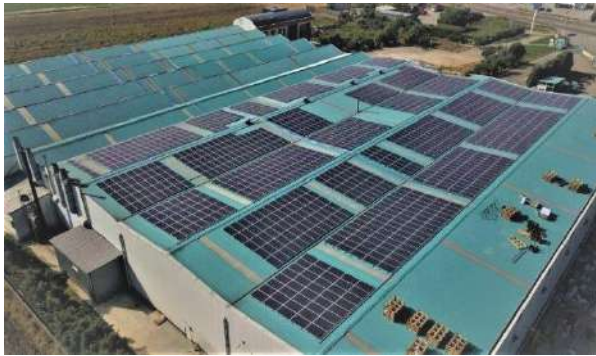
Yem- Tar Makine 480 kWp/400 kWe
